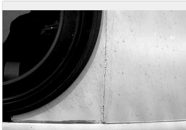
Bridging (paint failure as shown)
